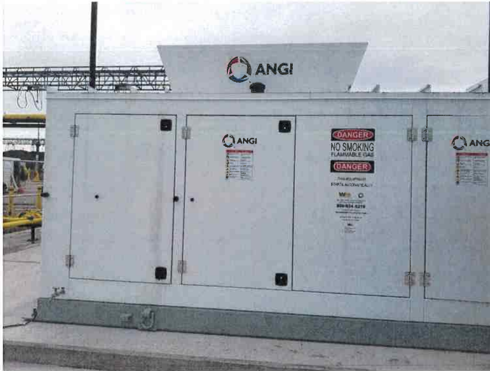
Figure 1: Typical Natural Gas Compressor
