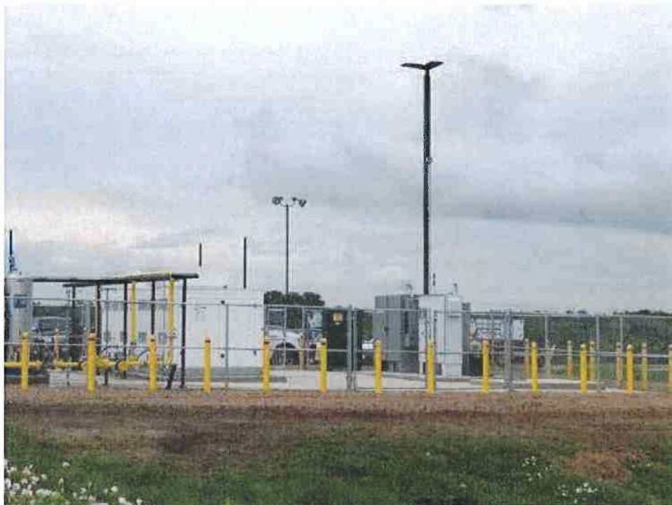
Figure 2: Typical Open-Air CNG Compound
