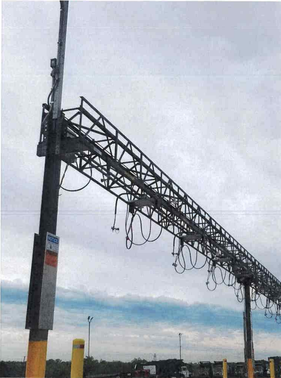
Figure 3: Typical Overhead CNG Fueling Truss
